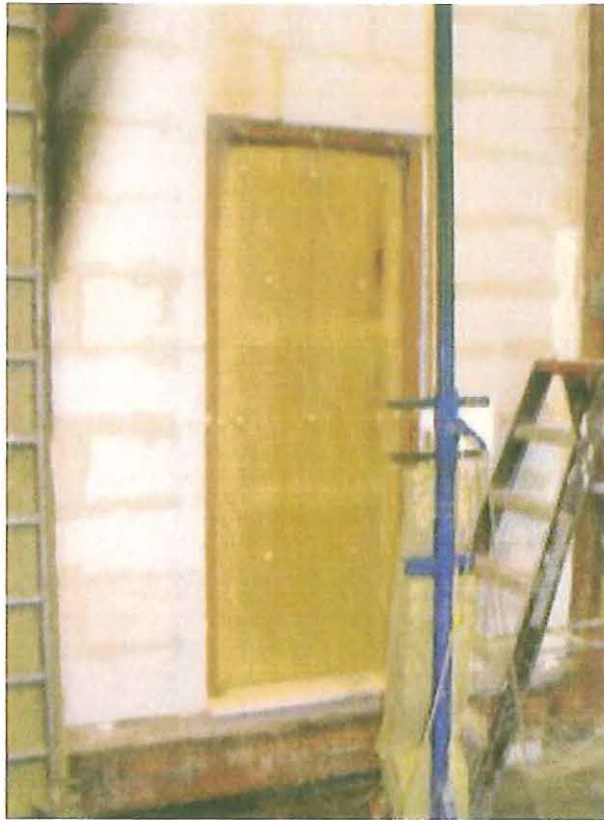
Photo 13: Pattern of insulation panels visible in door surface
